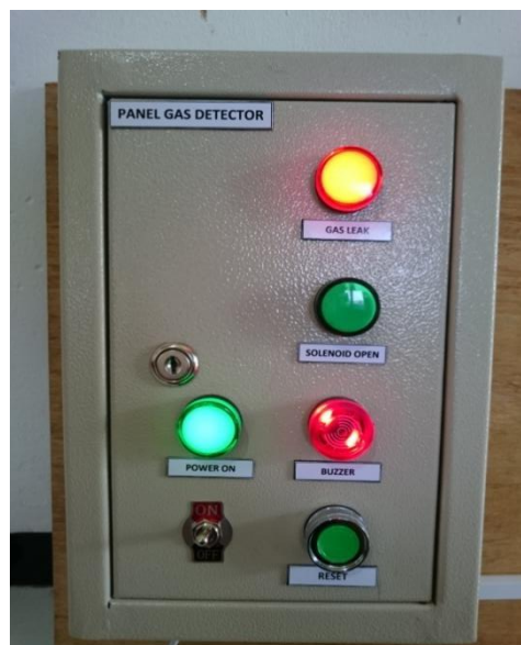
Gambar 9. Panel Gas Detector
